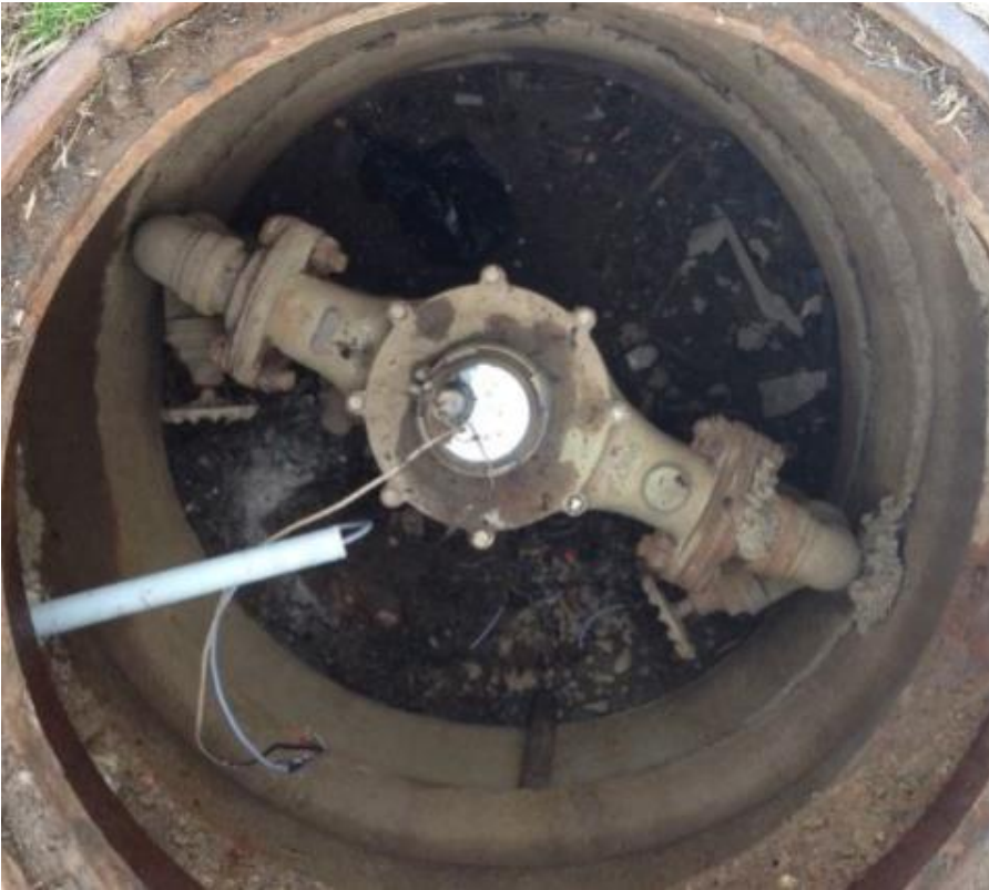
Before – with old gate valves
